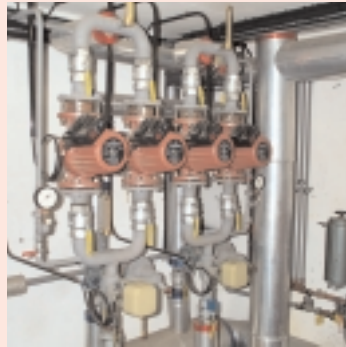
HVAC Control Systems
